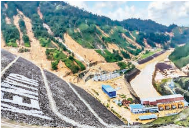
Kejadian fenomena aliran puing dan banjir lumpur di Tasik Kenyir yang menyebabkan kerosakan bangunan. The phenomenon of debris flows and mud floods in Kenyir Lake causing damage to buildings.
